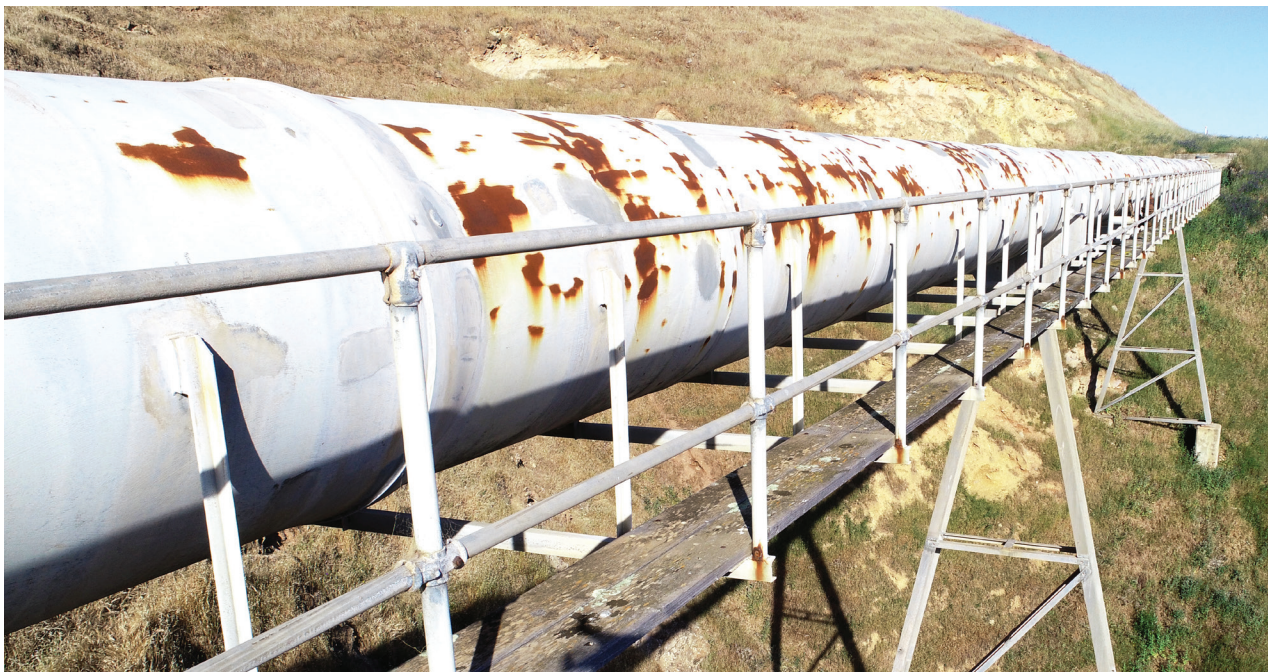
Corrosion and damage due to age degrades pipelines and increases the likelihood of ruptures occurring.
