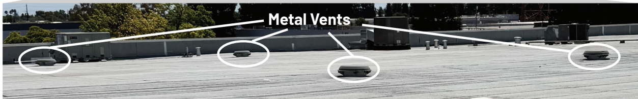
Building's Metal Vents
